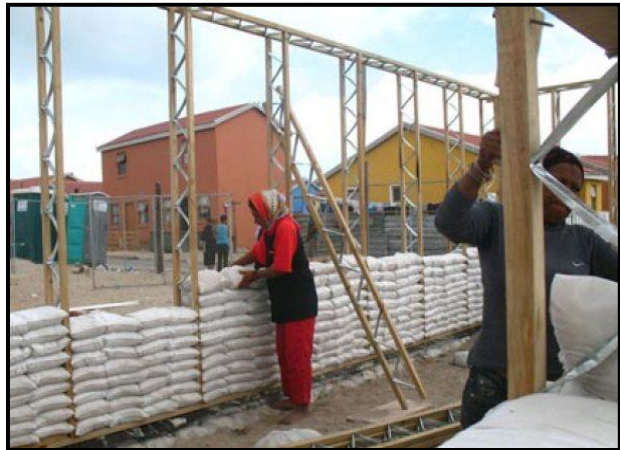
FIGURE 8c: Construction of a wall using wooden beams and sandbags, Sandbag Houses , Freedom Park, Cape Town, 2007.
